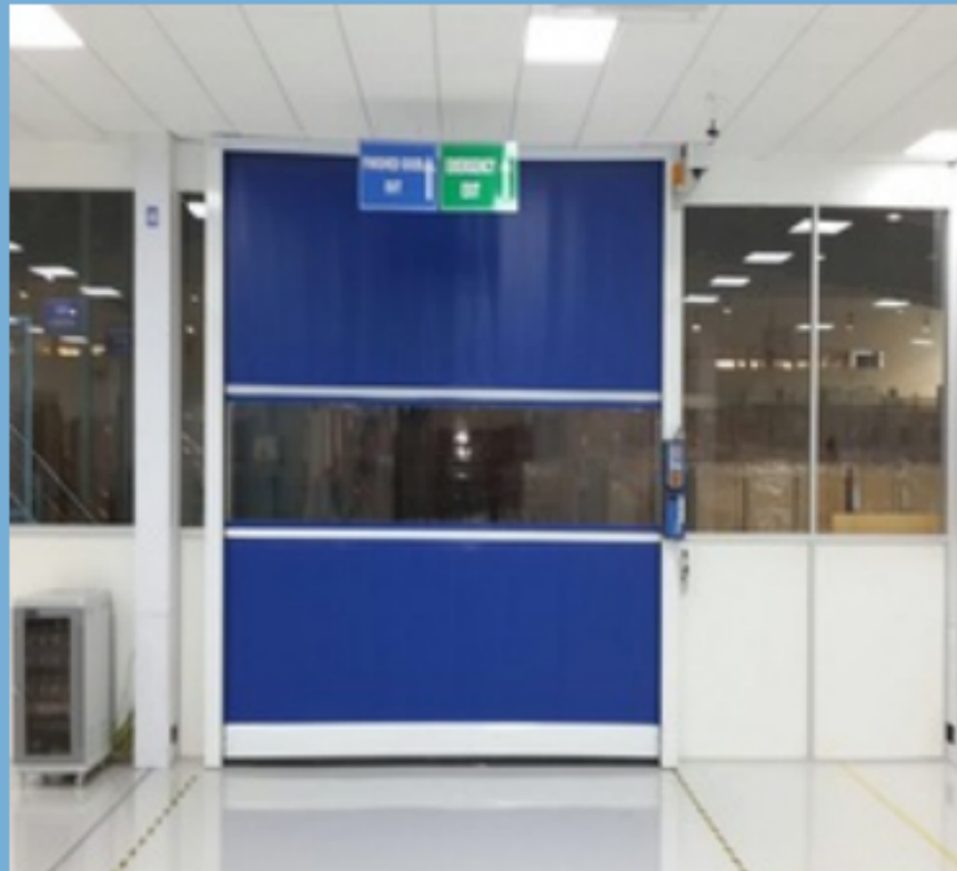
High Speed Doors In Clean Rooms
